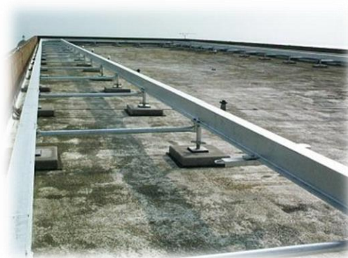
Steel track for BMU traversing
