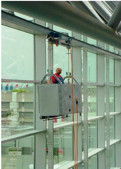
Monorail system – internal facade
